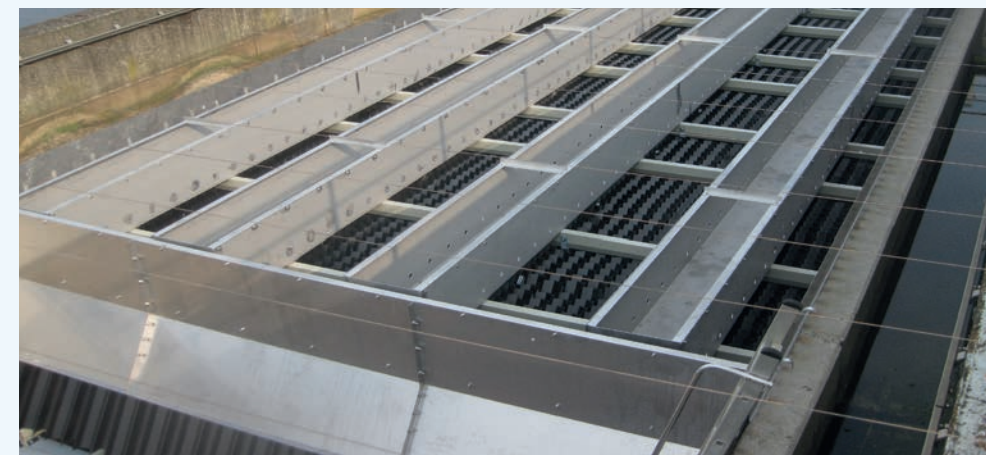
Secondary sedimentation tanks Activated sludge plant
