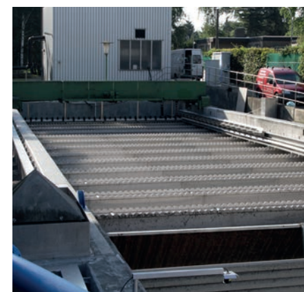
Rainwater treatment plant for 2m³/s
