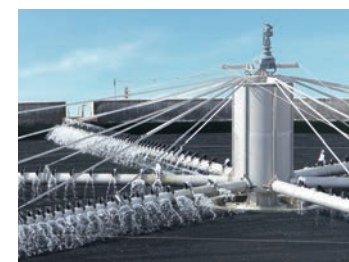
Biological water treatment
